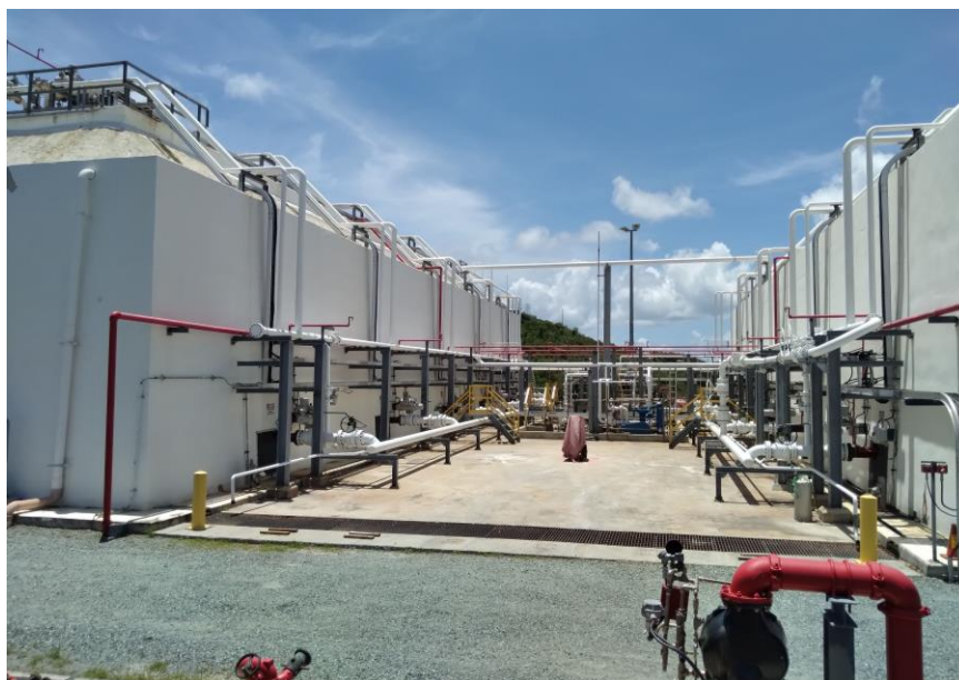
Figure 74 - Image of St. Thomas/St. John Propane Storage
