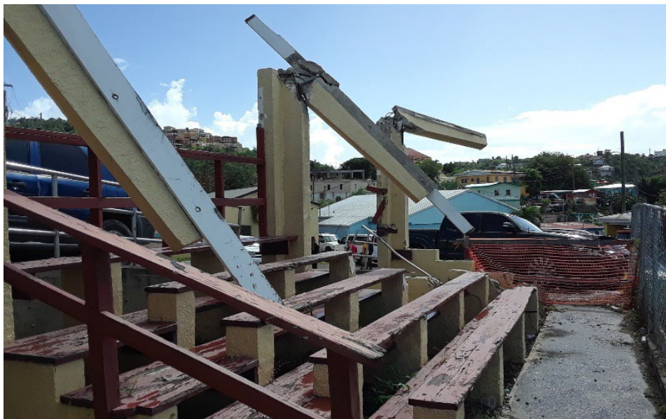
Pictured: Storm destruction on St. John near the school in Cruz Bay.
