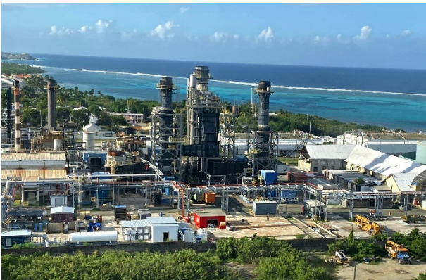
The USVI Water and Power Authority (WAPA), St. Croix, USVI. Photo Source: VI Consortium
