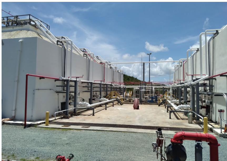
Figure 75 - Image of St. Thomas/St. John Propane Storage
