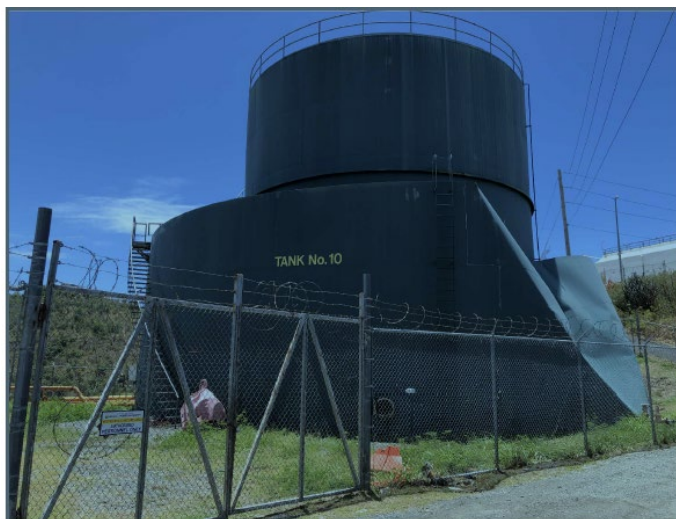
Figure 53 Illustration of Damage to Fuel Storage Tank No 10.
