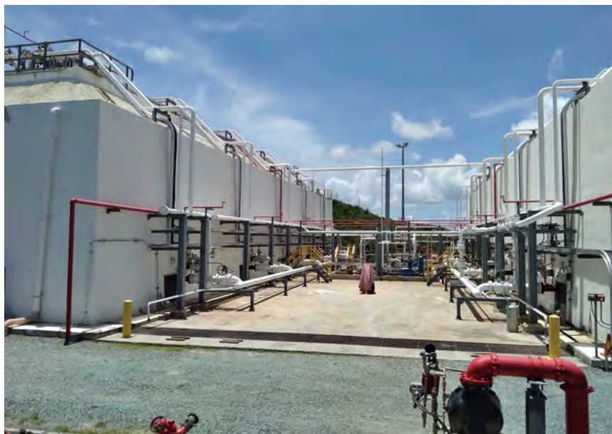
Figure 75 - Image of St. Thomas/St. John Propane Storage
