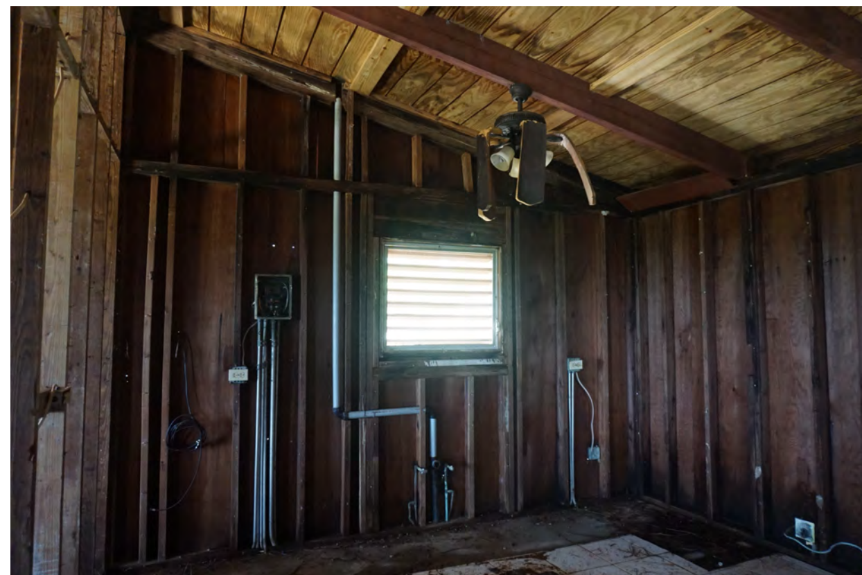
INTERIOR: ELECTRICAL PANEL REPLACE/ RELOCATE. REWIRE & REPLACE ALL OUTLETS & LIGHT FIXTURES WALL INTERIOR WALLS WERE STRIPPED OF DAMAGED PANELING
