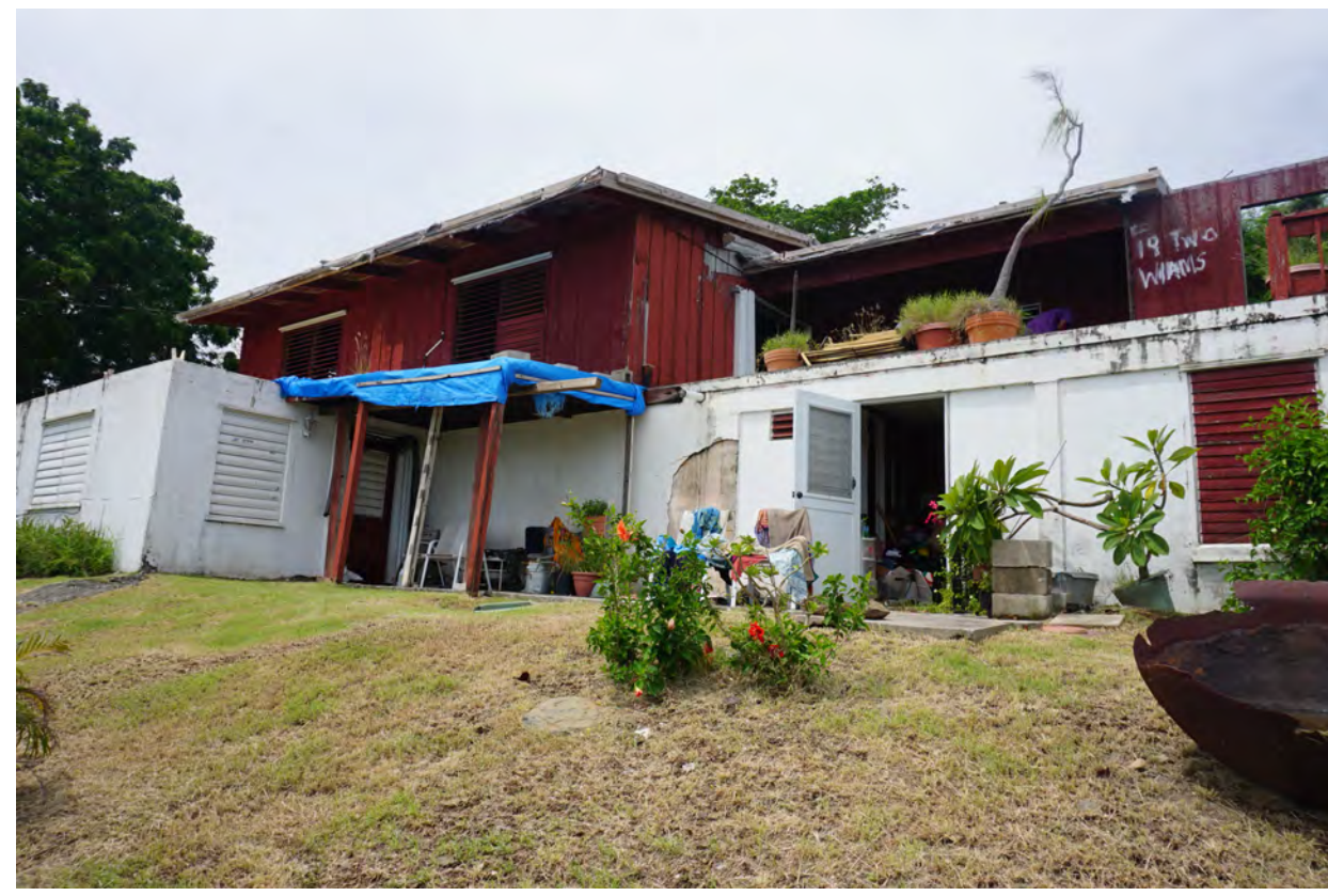
SOUTH SIDE LOST PATIO RAILINGS AND DAMAGED LOWER LEVEL CANOPY
