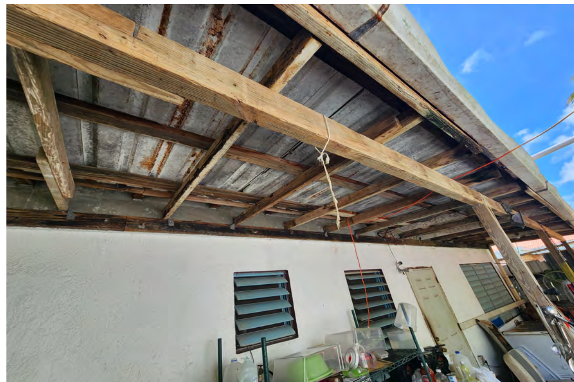
NORTH SIDE SHED ROOF DAMAGED, NON-CODE COMPLIANT SHED ROOF TO BE DEMOLISHED & REPLACED
