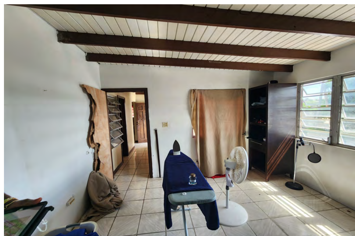
INTERIOR DOOR DAMAGE
