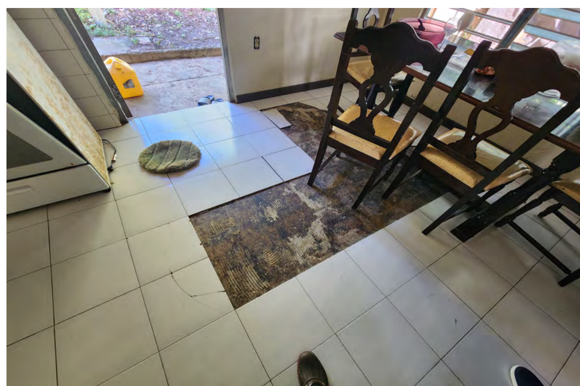
INTERIOR TILE DAMAGE
